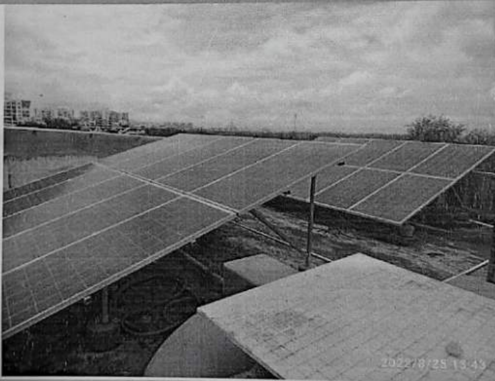
Solar Photovoltaic System- 15kWp
